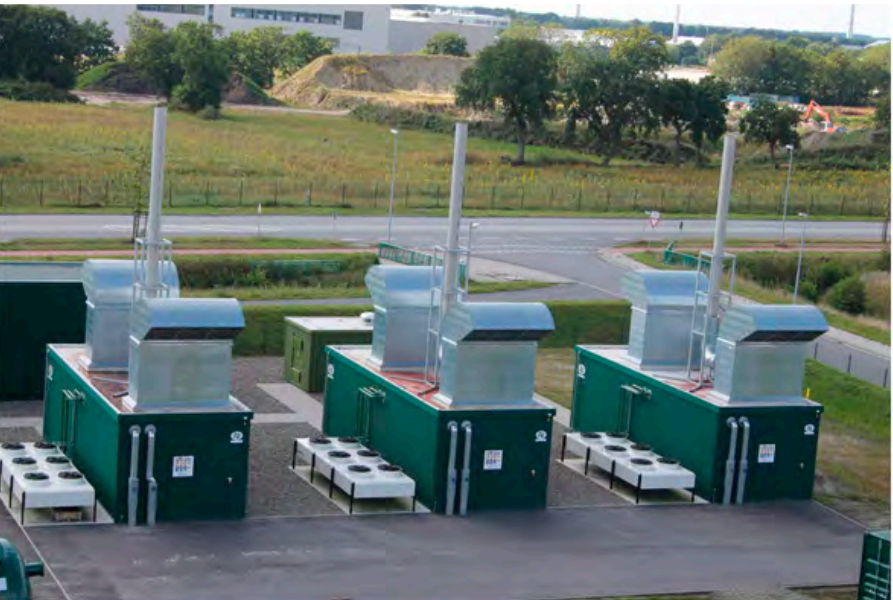
Figure A.55: CHP Generator
