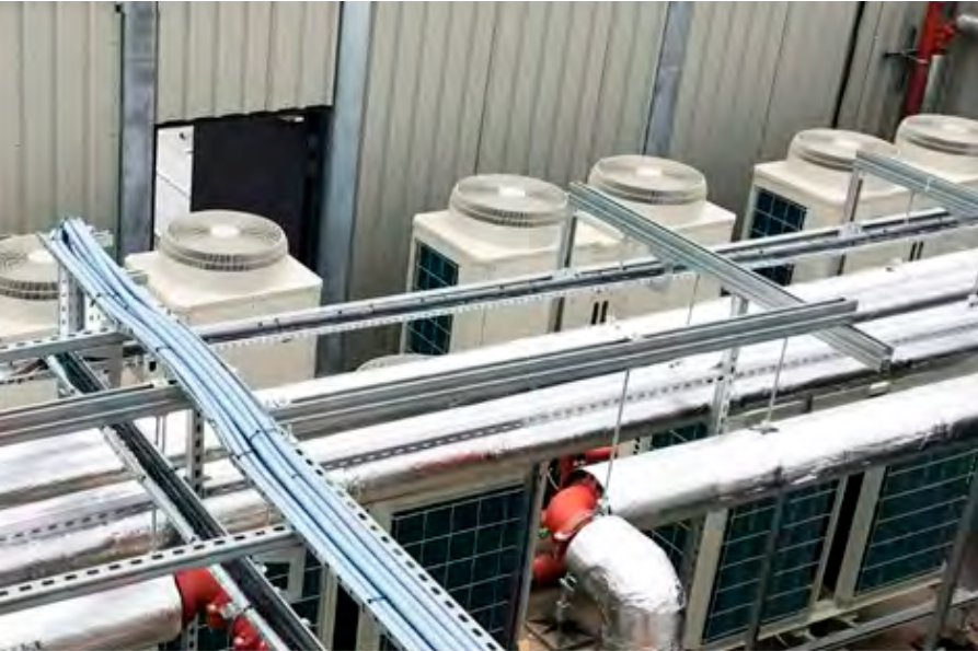
Figure A.56: Air Source Heat Pumps
